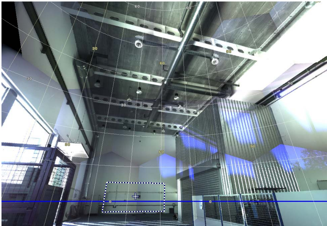
Figure 27: High-res 3D scanning (dotted square) of the MEP system example in the workshop area of CARTIF-3.
