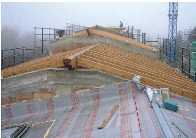
Laying of the breathable membrane straddles the ridge: overlapping the dotted line
