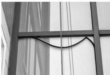
Figure 18: Loose gaskets or seals
