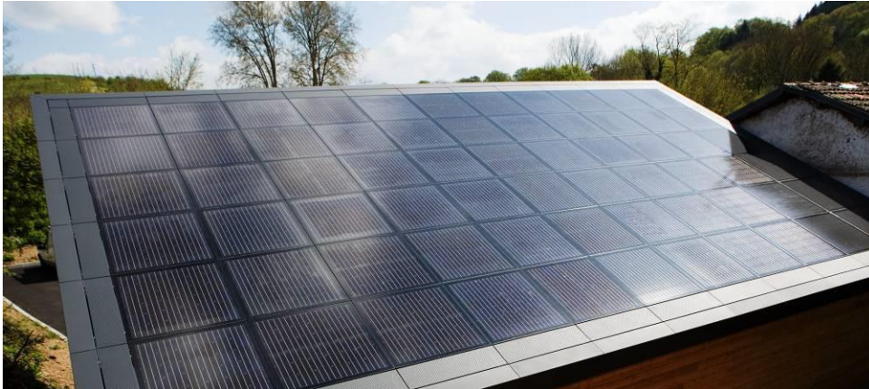
Photovoltaic panels installed on a roof
