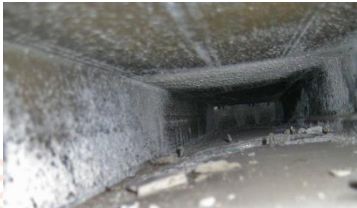
Construction waste/ dirt in ducts
