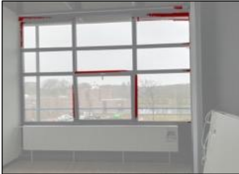
Figure 16: Visible image with leaks
