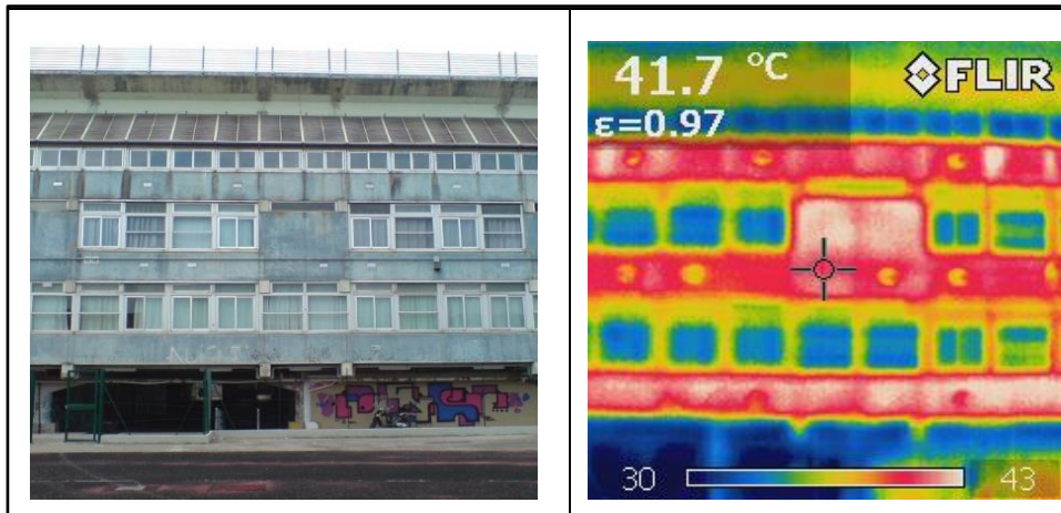
Figure 2: Example of a thermogram acquired in the East facade of the building
