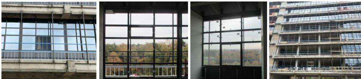
Figure 4: Outside and inside view of the façade system and its construction process
