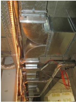
Figure 5: Photo from the Hogekamp facility showing the central duct system in the hallway. Critical are the right connection between duct parts and right installation of the suspension brackets.
