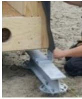
Figure 17: Reference photo from the mounting between the foundation-ground floor and the sealing
